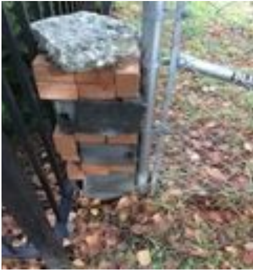
The gap in this fence has a provisional form of Access Control, it may be somewhat successful, but won't keep someone out who really wants in. It will also require constant attention to assure it is not disassembled.
