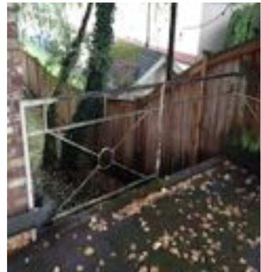
Missing fence pieces at Anderson Apartments, the side yard here shows evidence of use as a public toilet.
