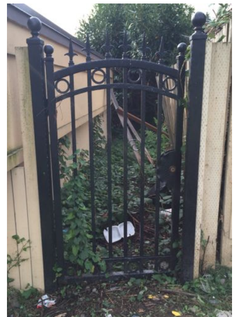
This gate behind Rainier Laundry could be an excellent example of good access control, however it seems that its lock is broken, or unused.
